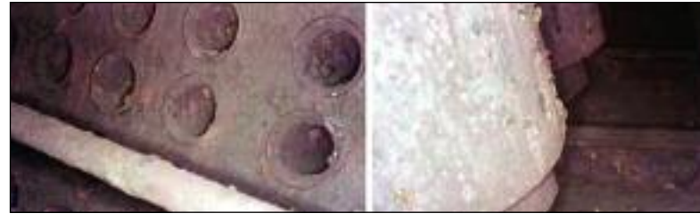
This image shows oxygen pitting in a boiler drum that was given inadequate layup protection. Courtesy: EPRI
