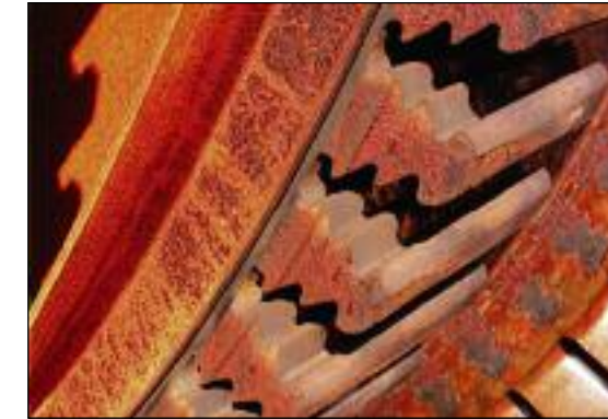
Deposits that contain chloride aggressively pit the turbine when it is allowed to sit in moist conditions. These pits become sites for corrosion fatigue. Courtesy: EPRI
